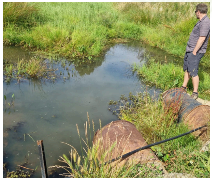
This structure posed a barrier to native fish migration and was identified for replacement as part of the Toitū Te Hākapupu restoration programme.
