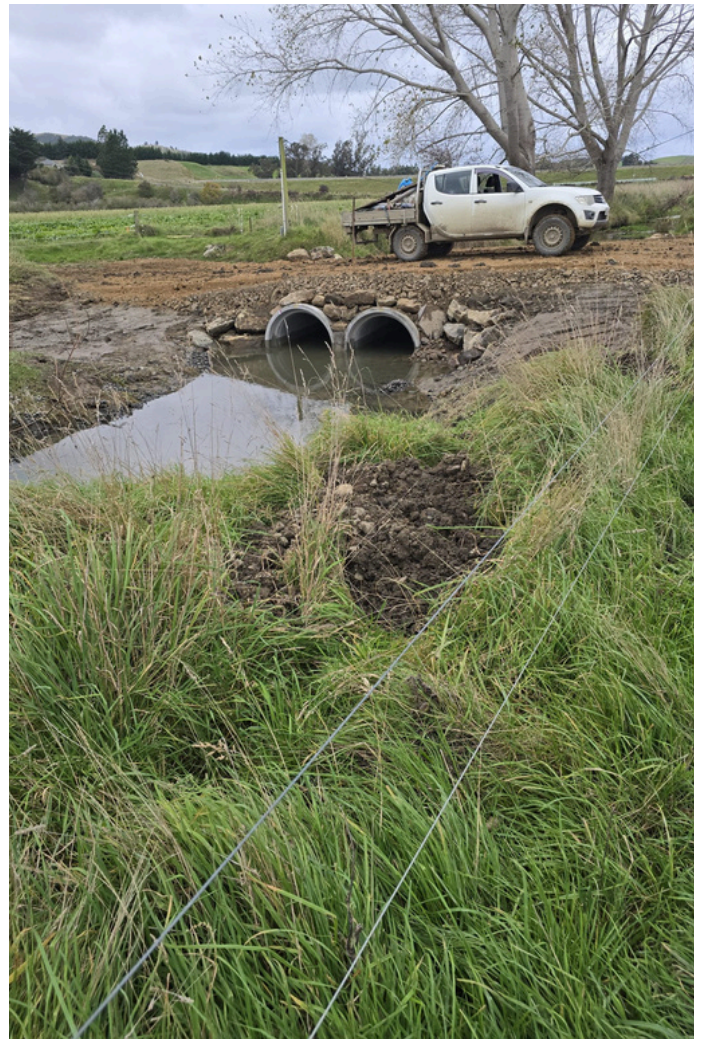
Twin 1200mm culvert installed at Watkin River, April 2025. This structure was delivered by Cargill Contracting Ltd for the Otago Regional Council.
