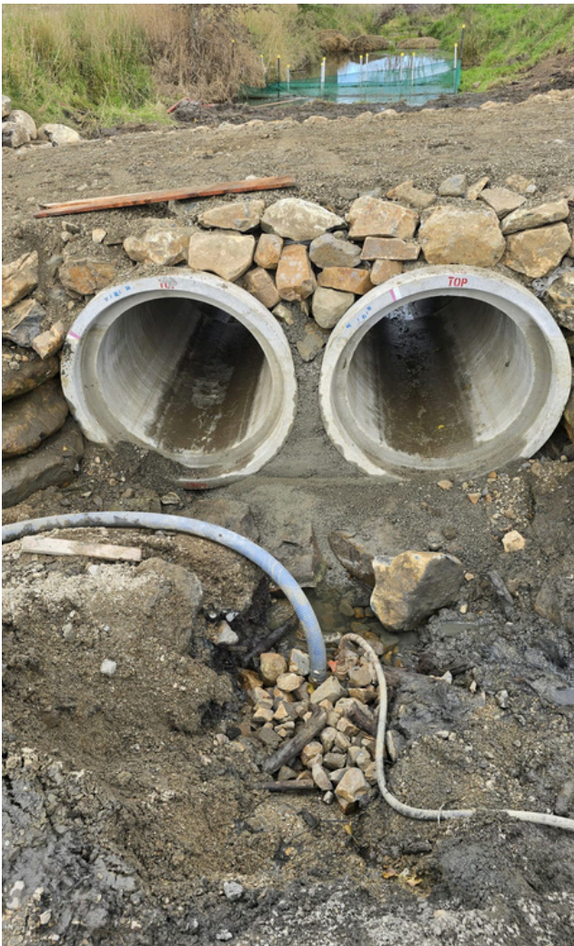
Installation of a twin 1200mm culvert with compacted rock bedding to support fish passage and resilient flood flow on the Watkin River, April 2025.
